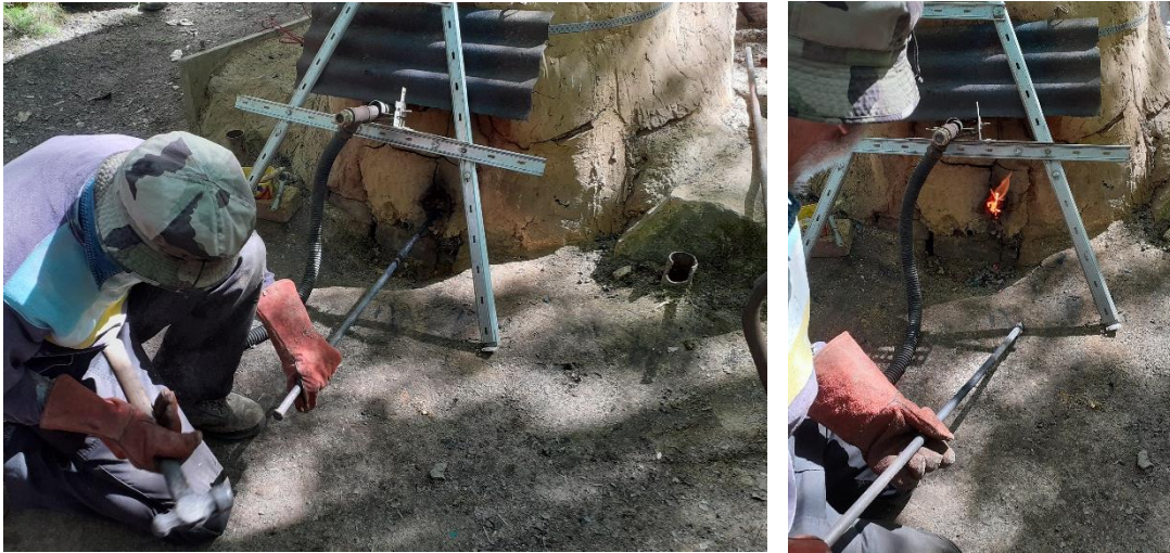
Figure 4.85 - Types 2 and 3: A boring stick is inserted through the tapping arch. (Author's image).
